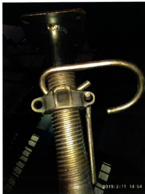
Fig. 4. A view of Collar nut and Pin failure
